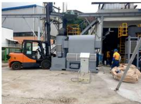
[small incinerator(100 kg/h)]
